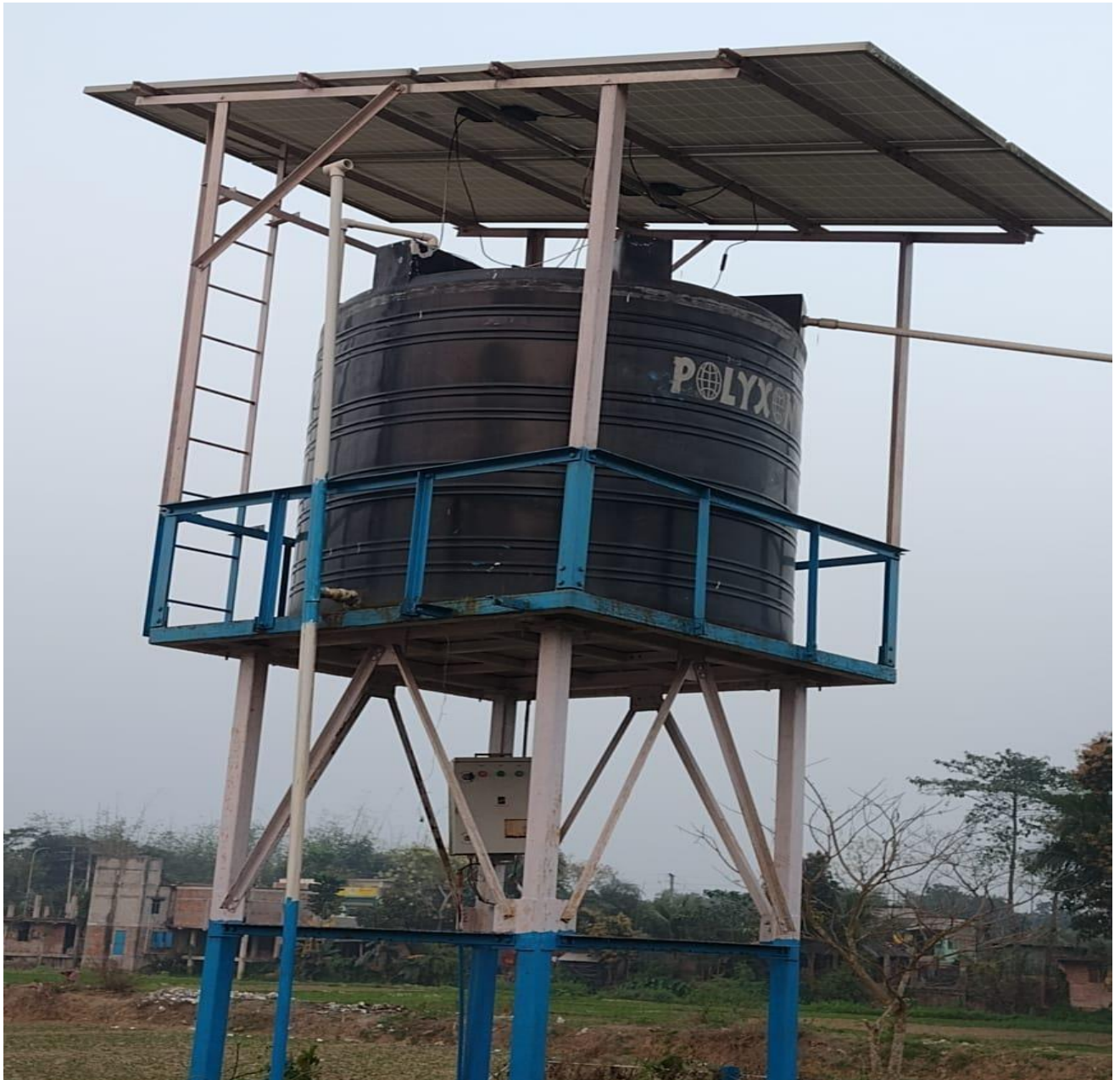
Figure 3: Solar power based backup water pump, Siddhinath Mahavidyalaya
